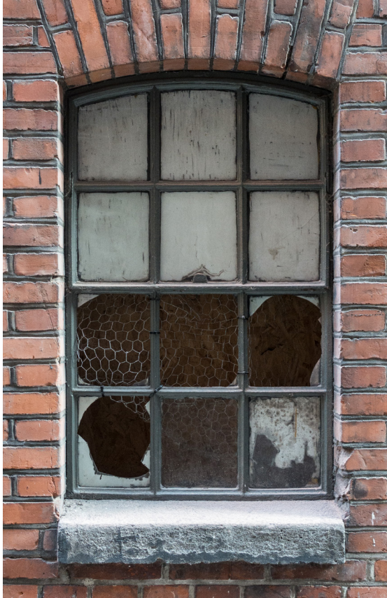
A devastated window in the alley. Multiple materials and textures and the passage of time create a complex scenario.
