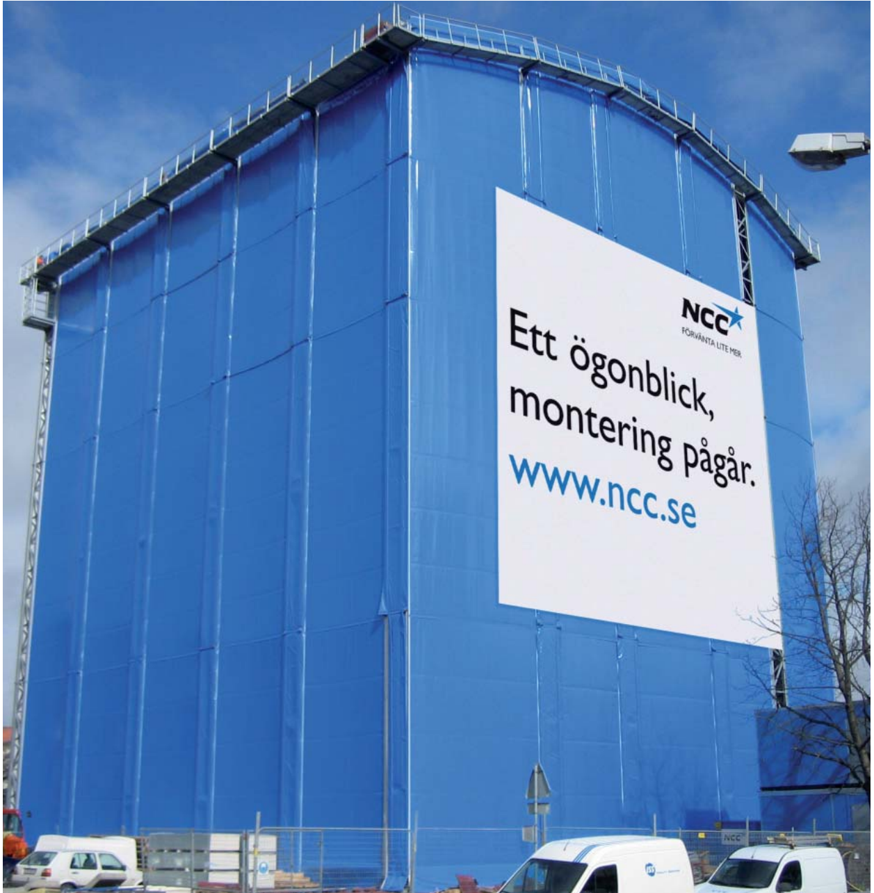
NCC Komplet construction site. 'One moment please, Assembly in progress'. Photo: NCC Komplet
