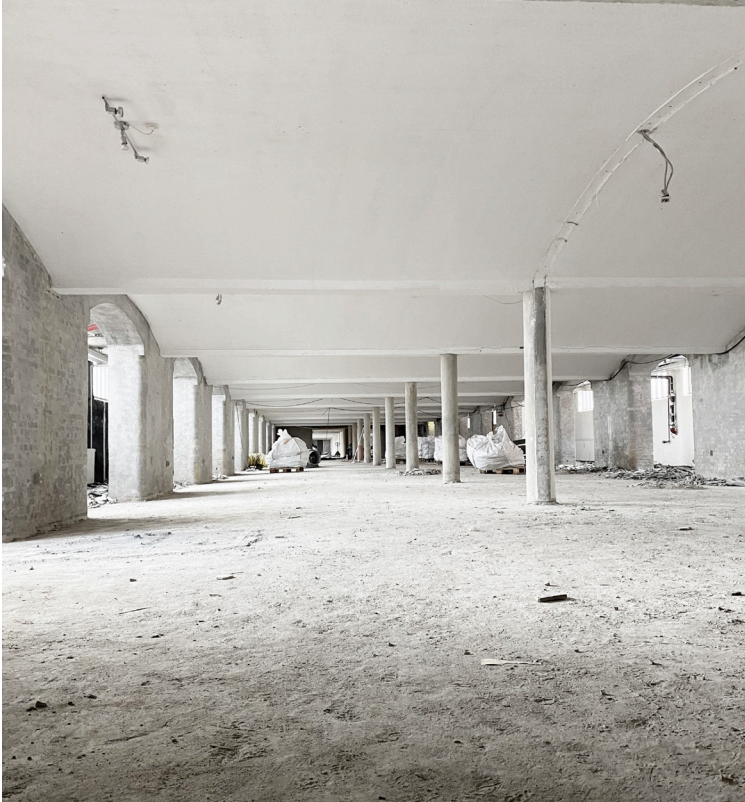
An empty part of the basement showing the centrally placed columns as a bearing element of the arched ceiling.
