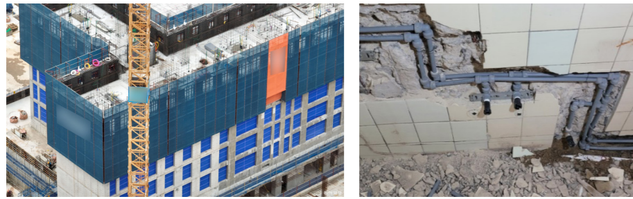
Fig05. Pipes embedded within the structure is not easily repairable and corrodes faster than concrete structures, thus shortening the lifespan of the building.
