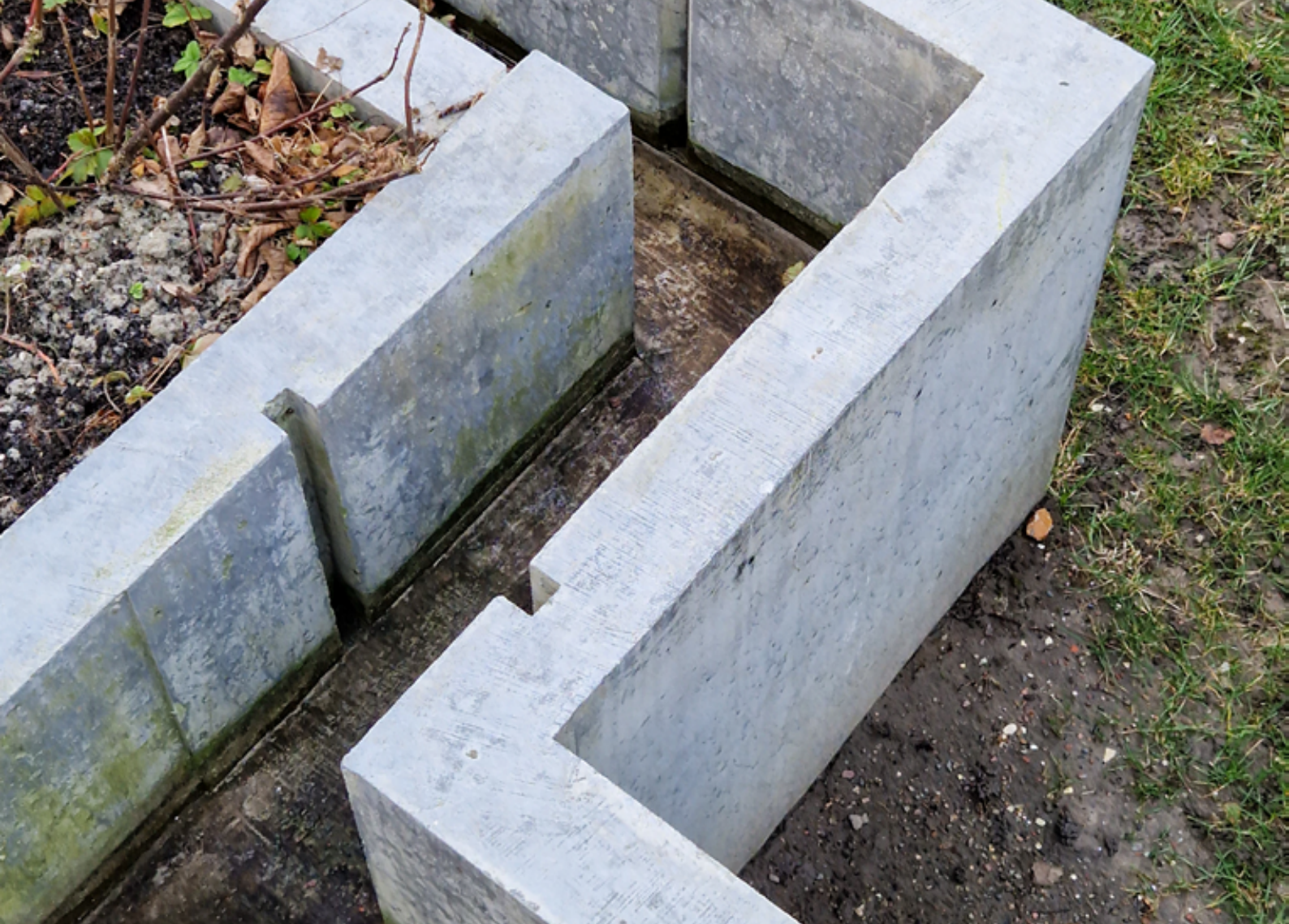
The concrete trench with incisions that allow for play and interaction at The Courtyard of the Future at Straussvej by BOGL, WSP, and Lendager (2021). photo by Emil Dencher, 2024.
