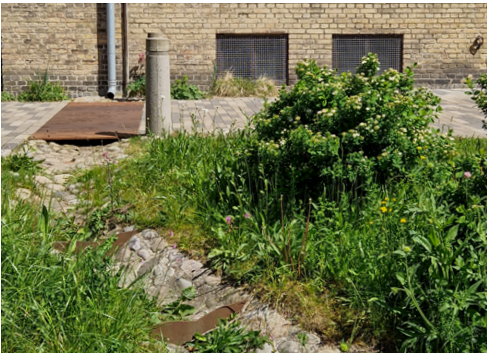
The trenches at The Courtyard of the Future at Askøgade, by Niels Lützen Landscape Architects, KUBEN Management, Labland, Envidan, and UiWE (2020). photo by Emil Dencher, 2024.
