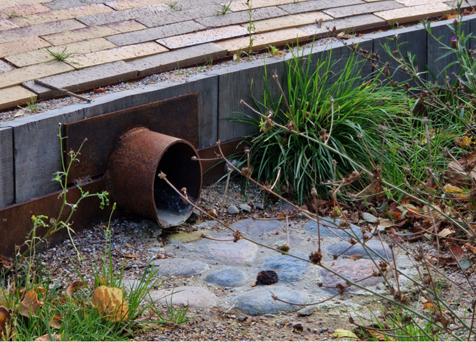
Outlet from one trench into another cobblestone trench at Karens Minde Aksen by Schønherr (2023). photo by Emil Dencher, 2024.
