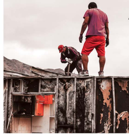
Campamento after Fire Accident Fig 12
